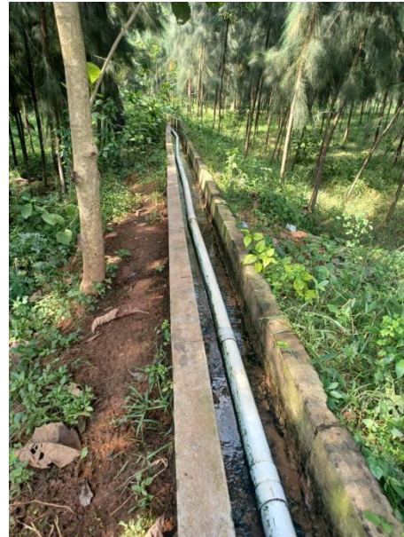
Pipeline carrying treated effluent to irrigation fields
