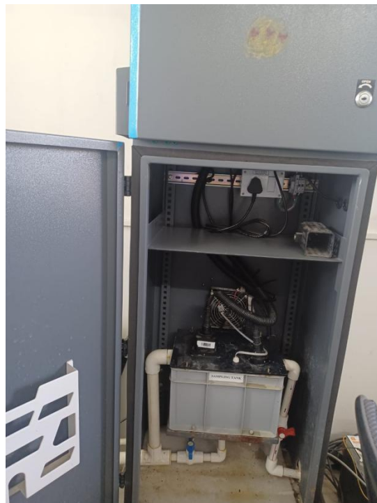
Online Continuous Effluent Monitoring System
