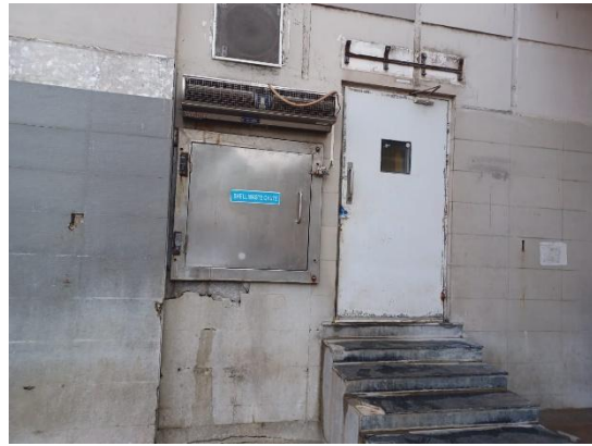
Cold storage for storing solid waste and solid waste chute
